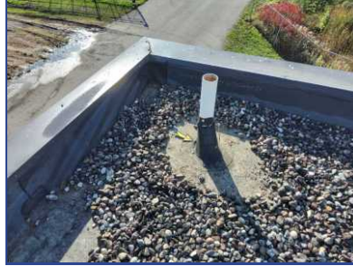
Need New Pipe Boot
