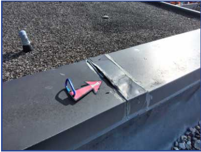
Sealant under metal cap deteriorated
