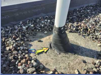
Need New Pipe Boot
