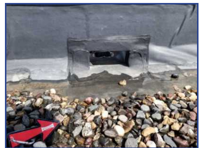
Section B - Def 1 - Before Photo
