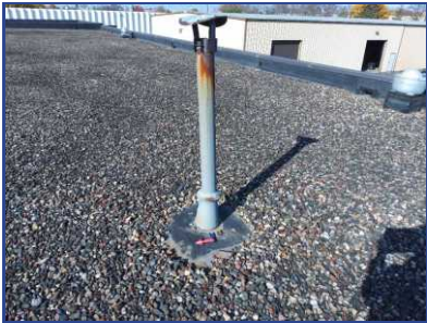
New target patch needed with new flashing
