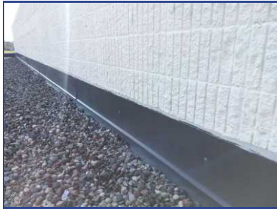
Metal sealant deteriorated
