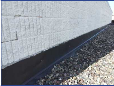
Metal sealant deteriorated
