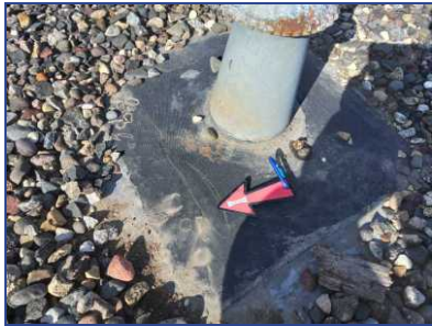
New target patch needed with new flashing
