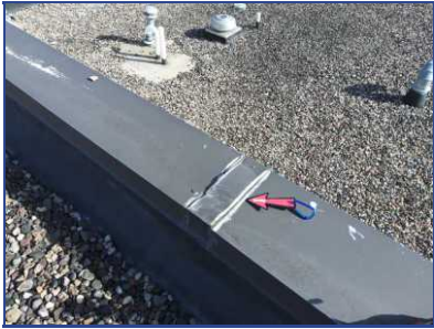
Sealant under metal cap deteriorated
