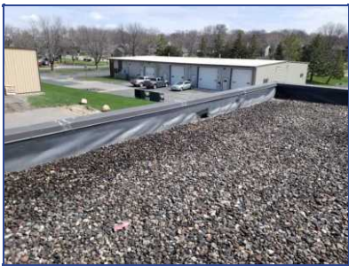
Section B - Def 3 - Before Photo
