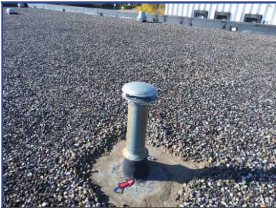
Membrane flashing voids, splits or open side laps
