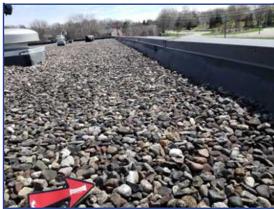
Section B - Def 3 - Before Photo
