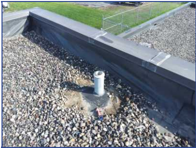
New target patch needed with new flashing
