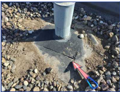
New target patch needed with new flashing
