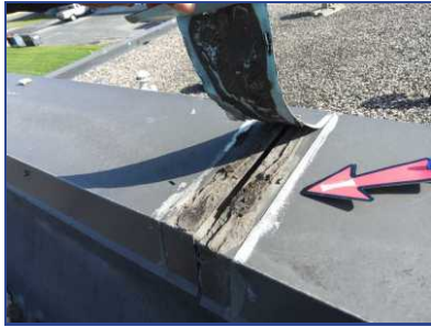
Sealant under metal cap deteriorated
