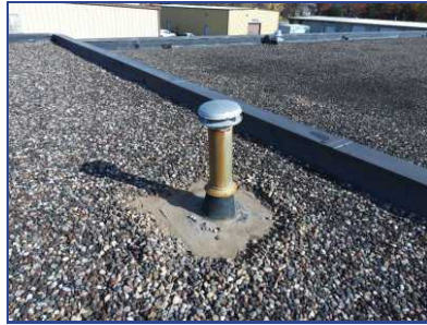
Corroded metal flashing
