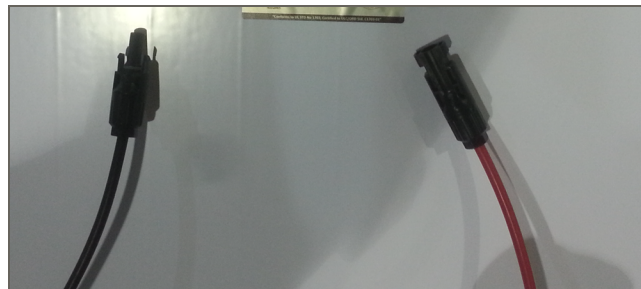
[Figure 20] Wires and connectors from the sign enclosure.
