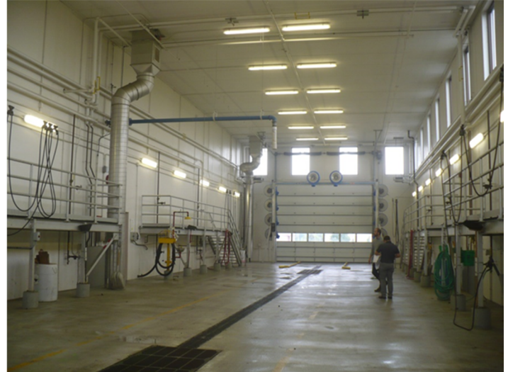
Above: Large wash bay
