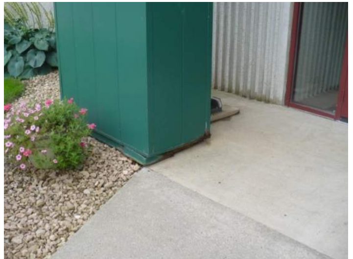
Above: Typical damage at base of the administration area
