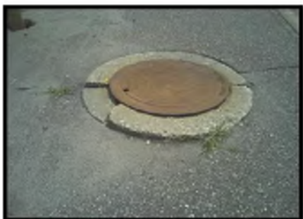
Traffic Signal Handhole
