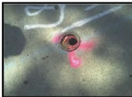
Water Gate Valve
